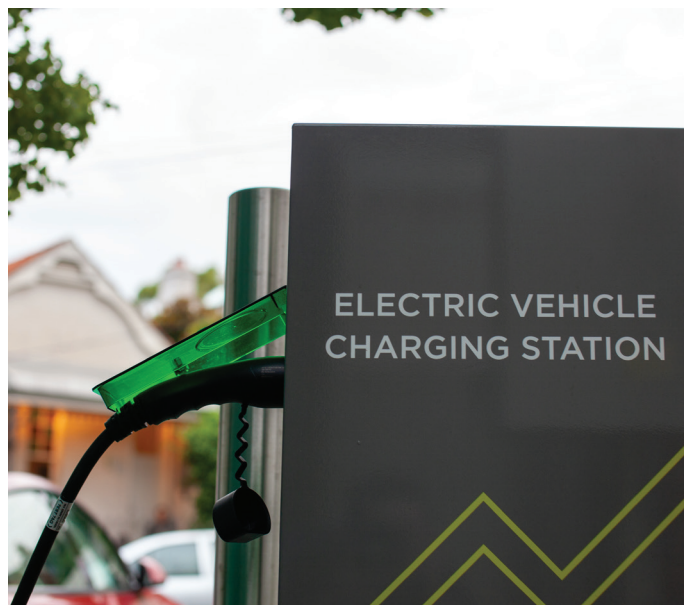
New electric vehicle charging station Goodhope Street, Paddington
