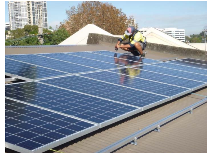
Solar PV System installed on Fletcher Street Depot.
