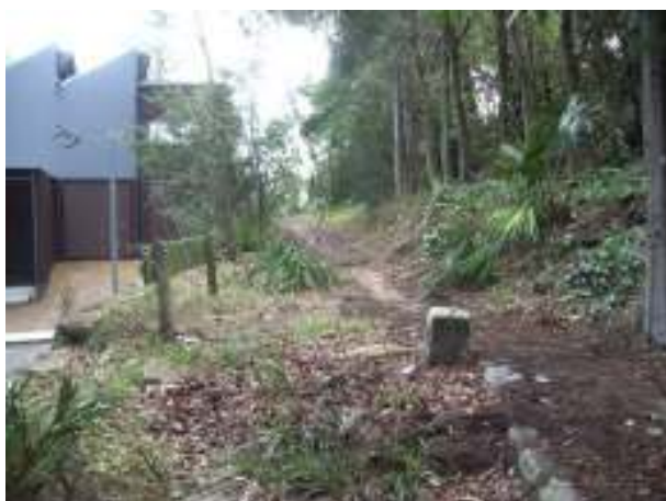
Photo 13 Obstructed overland flow path in Cecil Street
