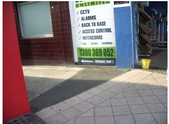
Photo 6: Worth Arcade draining ponding on New South Head Road, Rose Bay
