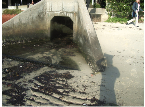
Photo 8: Stormwater outlet at Rose Bay
