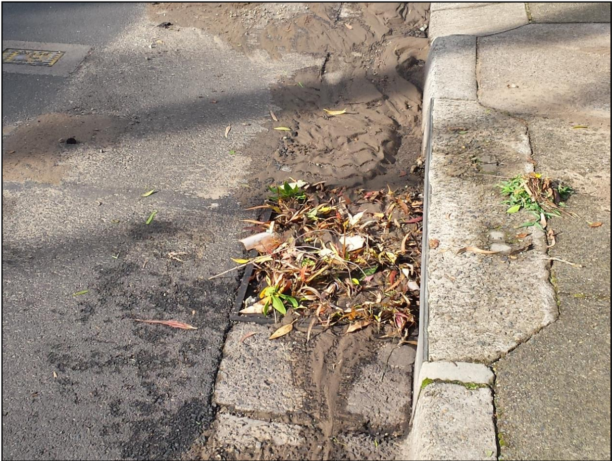
Plate 16 View showing blockage of a stormwater pit located on Glenmore Road following a storm event in 2015
