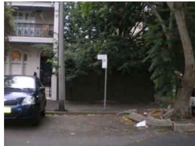
114. Ground Floor Inundation Property on Sutherland St with inundation reported. Walls could offer protection to some extent
