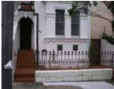
173 Windsor St Above floor level inundation
