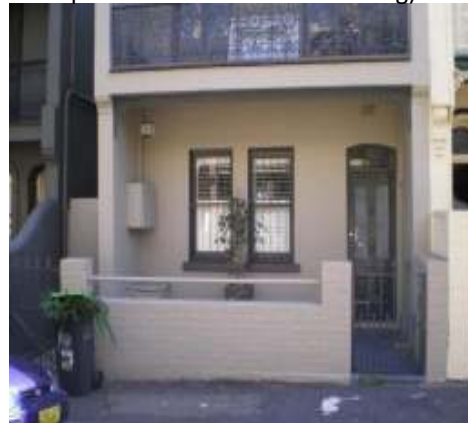
121 Underwood St Rising groundwater causes inundation of the basement during major storm events.
