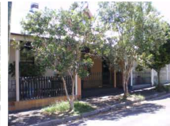
36. Ground Floor Inundation or Floor Below Road Properties on Harris St with above floor level inundation recorded. Flow most likely from rear end (Sutherland Ave)
