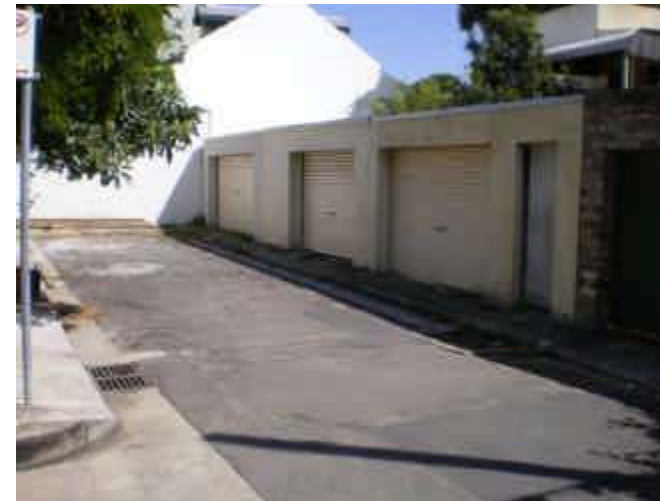
83. No Flow Path Ponding in Ashton Lane
