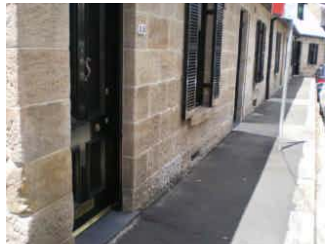
82. Ground Floor Inundation Properties at risk of being inundated on Underwood St.
