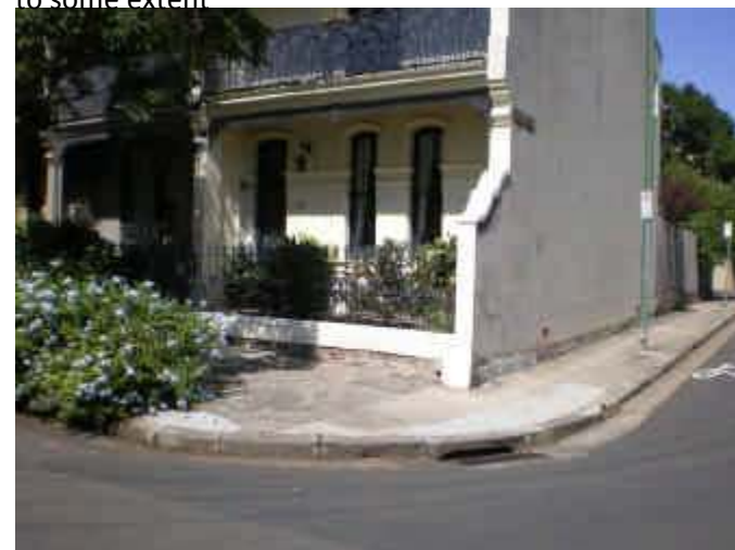
118. Ponding & Ground Floor Inundation Ponding at the end of Hopetoun St
