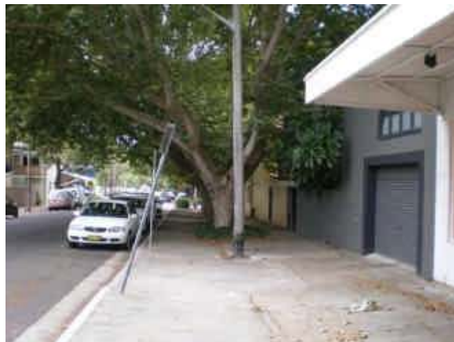
71. Ponding Footpath lower than road
