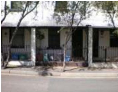
184 Underwood St Above floor flooding due to a drainage problem
