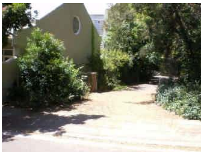
33. Flow Diversion Possible flow path off the lower most part of Harris Street
