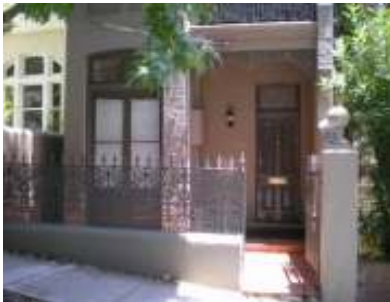
280 Glenmore Rd Groundwater seepage due to storm events.
