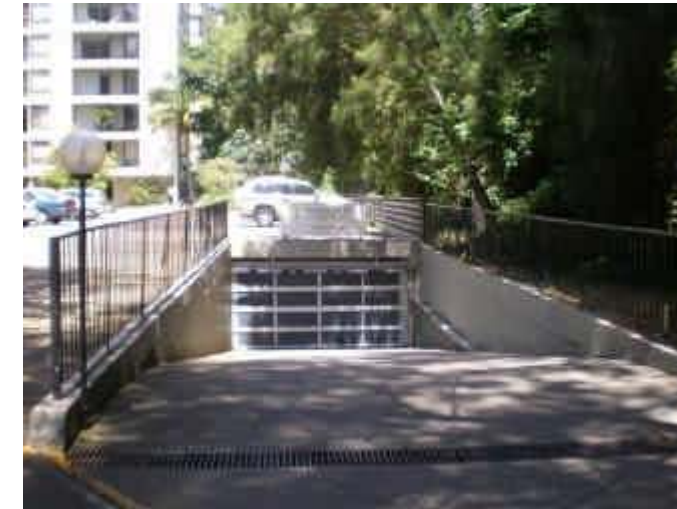
111. Garage Below Road Another garage on Hampden Street at risk of being inundated.
