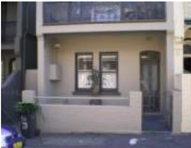
121 Underwood St Rising groundwater causes inundation of the basement during major storm events.
