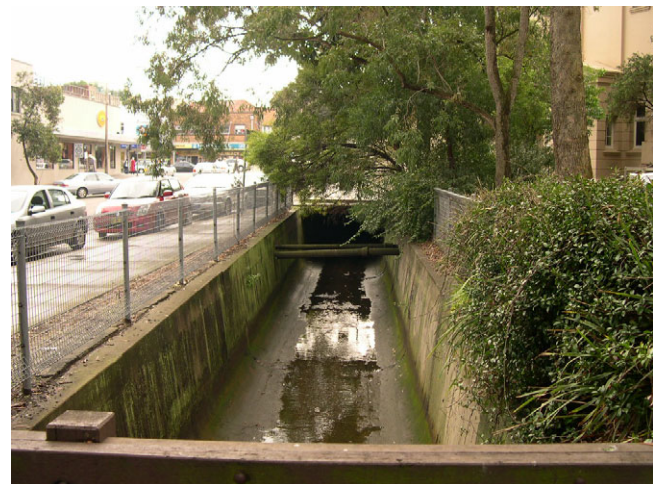
Figure 5: Open channel next to Kiaora Road. The FRMS will consider the propensity for drains to block and measures to avert blockage.
