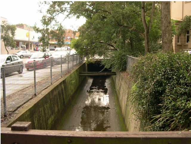
Open channel next to Kiaora Road. One recommendation is to replace the existing fencing next to the channel with structurally designed safety fencing, to reduce the potential for large objects—including motor vehicles—from blocking critical culverts during flooding.
