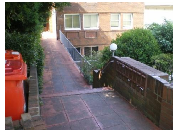
217. 103A Birriga Road Problem identified by Reference 2, field trip results show: Garage below road, Flooding due to overland flow from road above property
