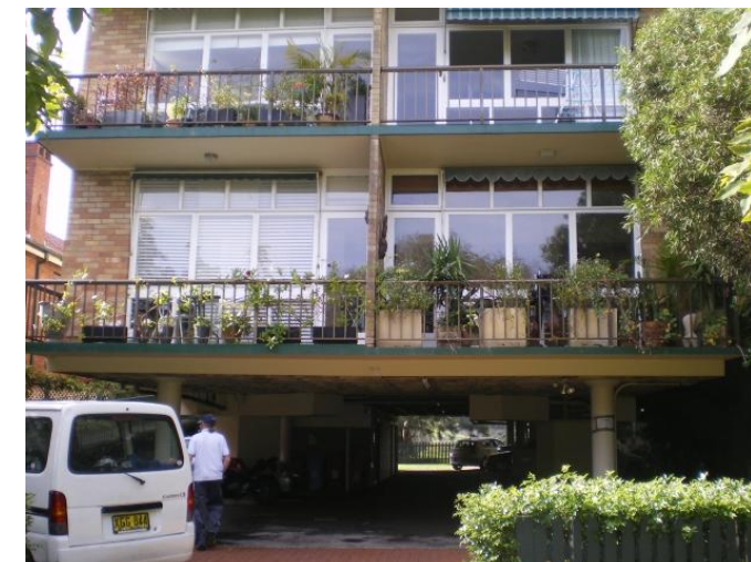
25. 22 Manion Avenue Problem identified by Reference 3, field trip results show: Street flooding reported, no problem identified
