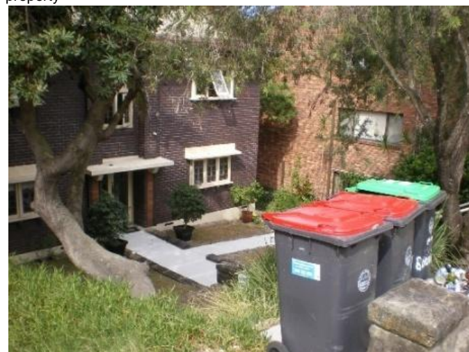
160. 53 Boronia Road Problem identified by Reference 2, field trip results show: Floor below road, Ponding on street, Flooding due to overland flow from road above property
