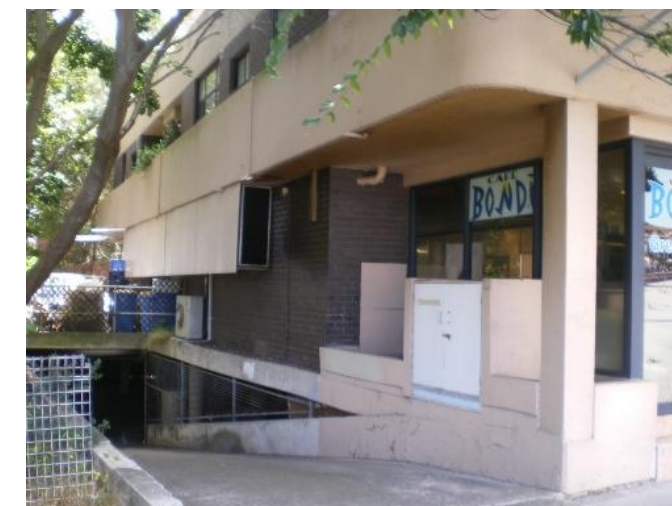
233. 624B New South Head Road Problem identified by Reference 2, field trip results show: Floor below road
