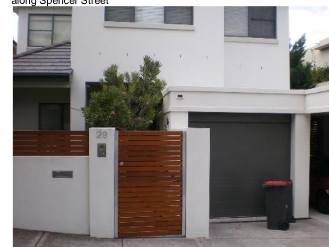
296. 29 Spencer Street Problem identified by Reference 4, field trip results show: Floor below road, Garage below road, High Flow along Spencer Street
