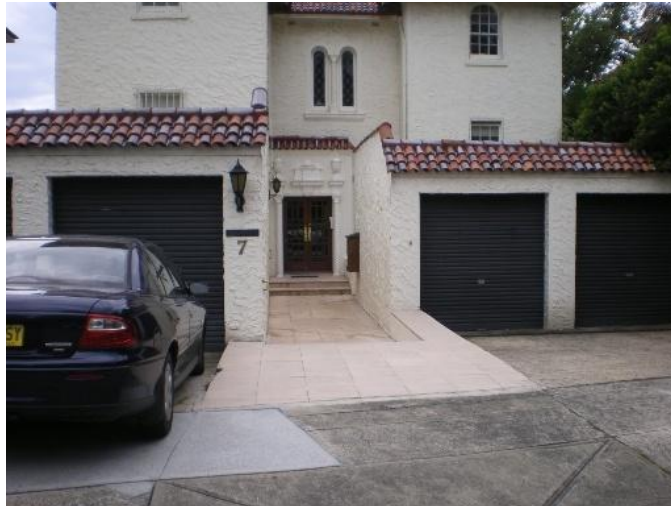
0. 7 Aston PL Problem identified by Reference 4, field trip results show: Floor below road, Ponding on street, Flooding due to overland flow from road above property
