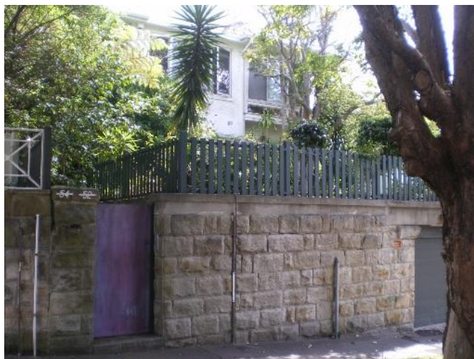
45. 52 Beresford Road Problem identified by Reference 4, field trip results show: Flooding due to overland flow from road above property
