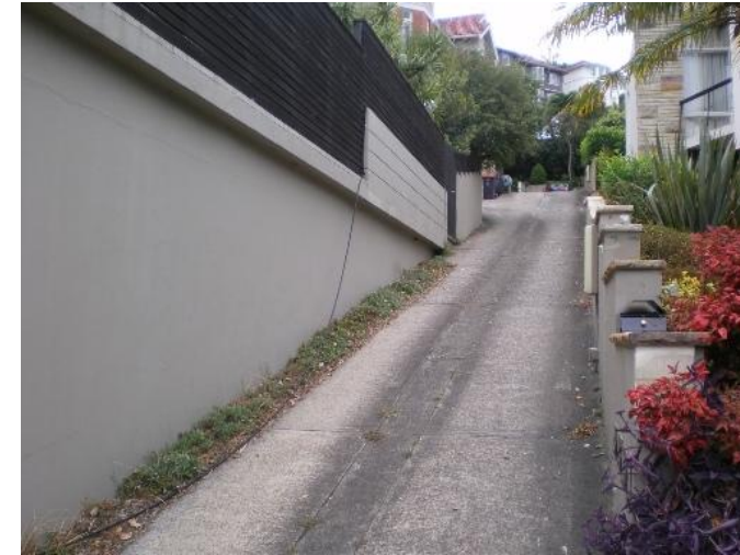
4. 13 Cranbrook Road Problem identified by Reference 4, field trip results show: Flooding due to overland flow from road above property
