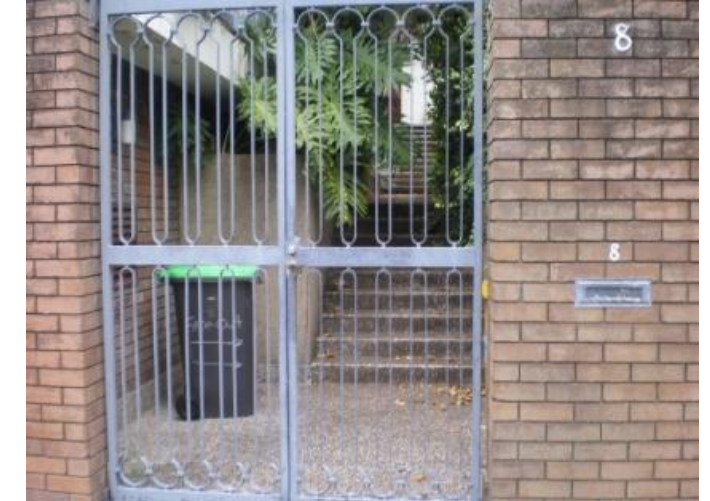
181. 8 Blaxland Road Problem identified by Reference 4, field trip results show: Floor below road, Garage below road, High velocity flow, Flooding due to overland flow path from adjacent street
