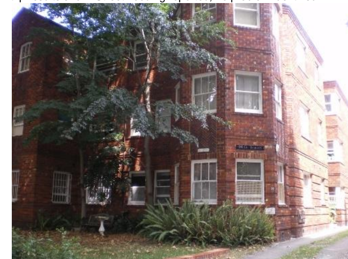
36. 24 Balfour Road Problem identified by Reference 2, field trip results show: No problem identified
