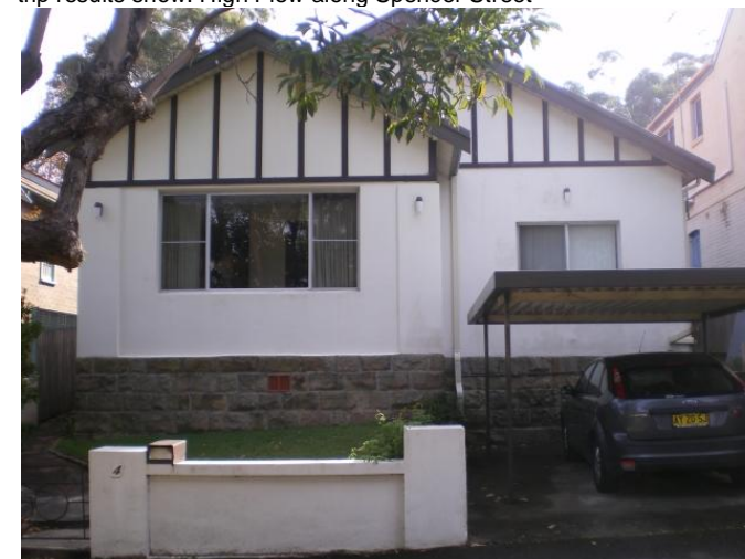
282. 4 Spencer Street Problem identified by Reference 4, field trip results show: High Flow along Spencer Street
