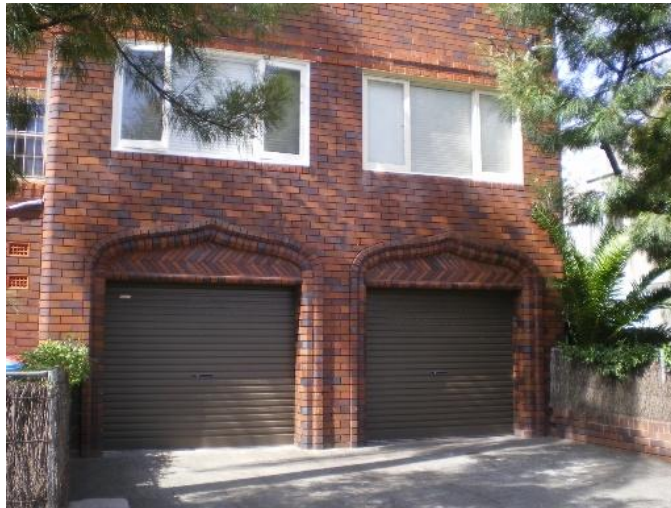
316. 34 Dover Road Problem identified by Reference 4, field trip results show: Flooding due to overland flow from road above property, Ponding on street
