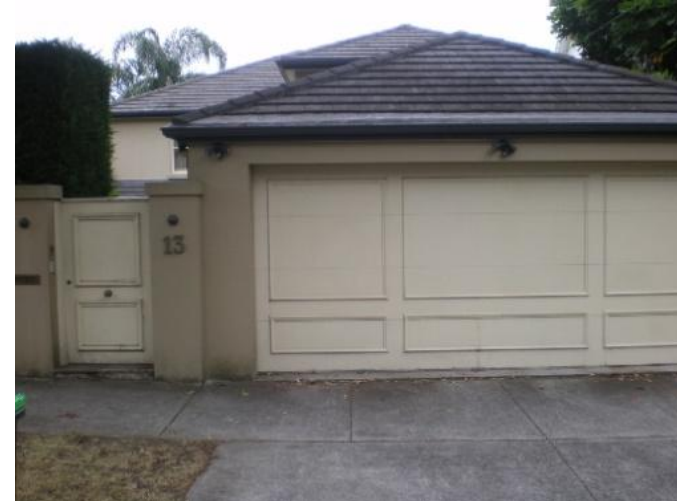
177. 13 Bundarra Road Problem identified by Reference 2, field trip results show: Floor below road, Garage below road, Ponding on street, Flooding due to overland flow from road above property
