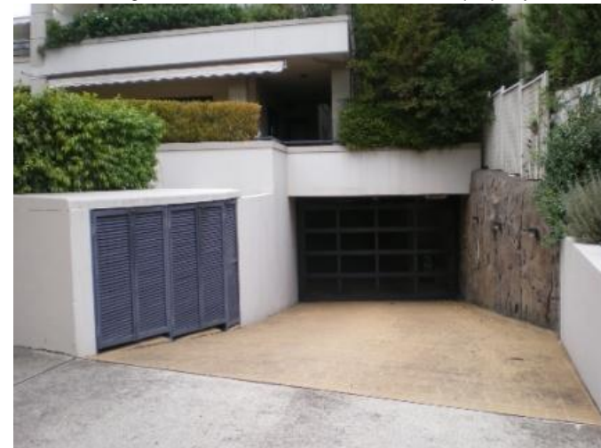
183. 12 Blaxland Road Problem identified by Reference 4, field trip results show: Floor below road, Garage below road, High velocity flow, Flooding due to overland flow path from adjacent street
