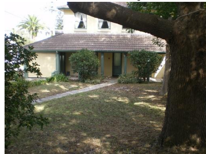
265. 2 Ebsworth Road Problem identified by Reference 2, field trip results show: Floor below road, Road and footpath graded towards residence, Main flow channel bordering residence
