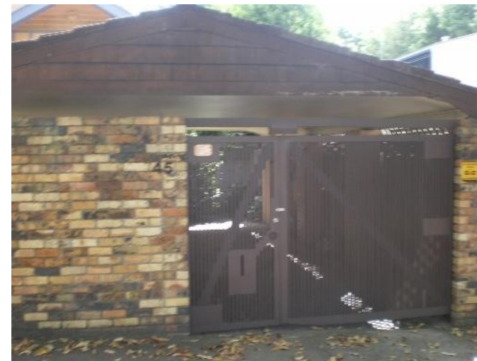
71. 45 Salisbury Road Problem identified by Reference 2, field trip results show: Garage below road, Main flow channel bordering residence
