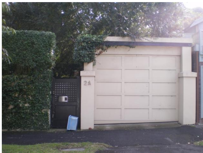
284. 2A Spencer Street Problem identified by Reference 4, field trip results show: High Flow along Spencer Street
