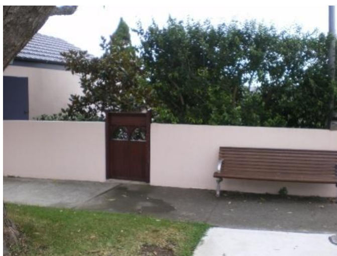
169. 19 Bunyula Road Problem identified by Reference 4, field trip results show: No problem identified
