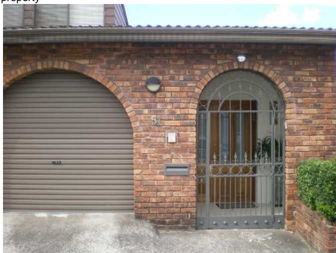
159. 51 Boronia Road Problem identified by Reference 2, field trip results show: Floor below road, Ponding on street, Flooding due to overland flow from road above property
