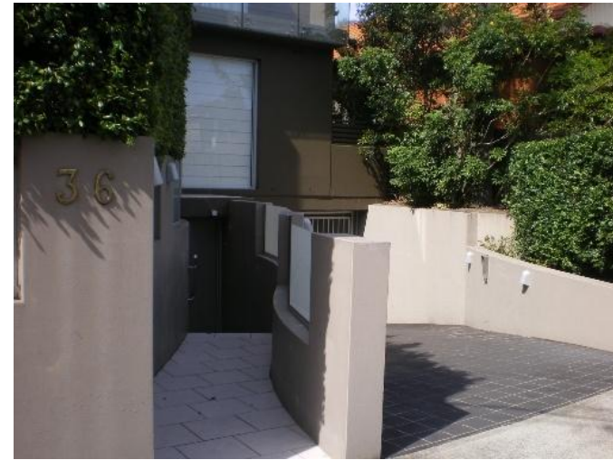
317. 36 Dover Road Problem identified by Reference 2, field trip results show: Floor below road, Garage below road, Flooding due to overland flow from road above property, Ponding on street
