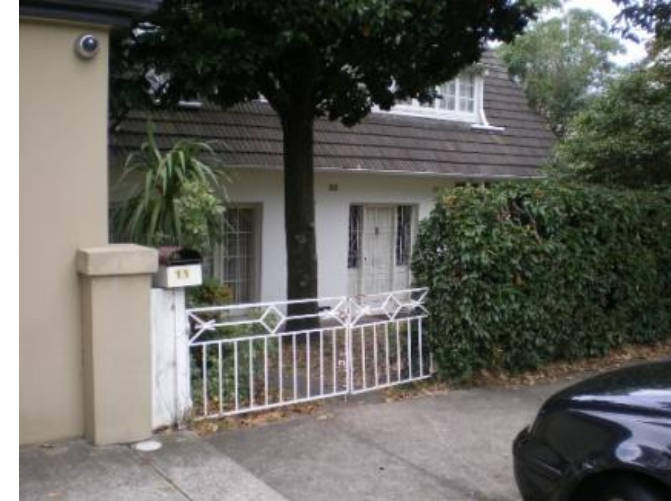
178. 11 Bundarra Road Problem identified by Reference 2, field trip results show: Floor below road, Garage below road, Ponding on street, Flooding due to overland flow from road above property
