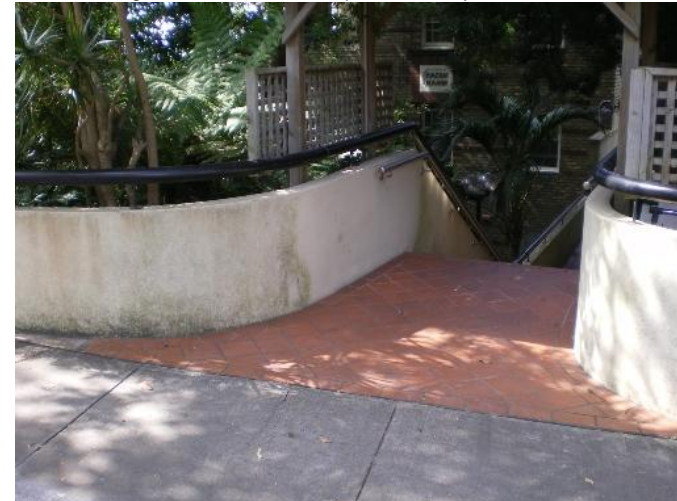
196. 94 Birriga Road Problem identified by Reference 2, field trip results show: Floor below road, Main flow channel bordering residence
