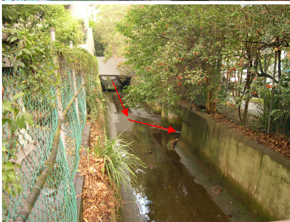
c. "Bifurcation" culvert entrance adjacent to Kiaora Road (on right, looking upstream)
