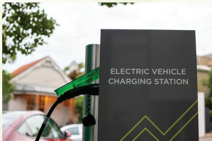
New electric vehicle charging station Goodhope Street, Paddington
