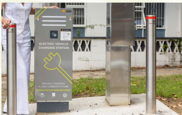
EV Charger at Birriga Road, Bellevue Hill
