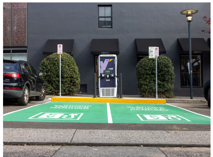
Electric Vehicle Charging Station at Dorhauer Lane
