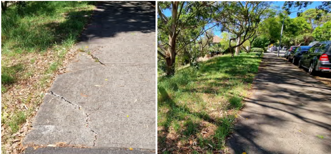
Figure 16 Tension cracks on footpath along Cranbrook Road
