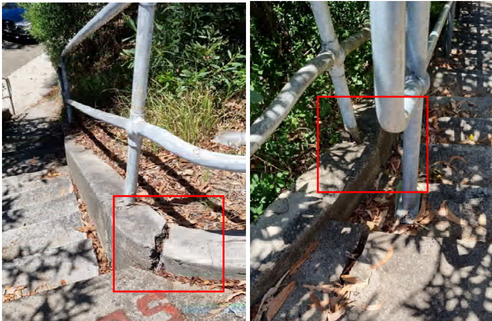
Figure 18 Cracked hand-rail kerb along an external stair.
