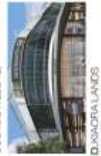
C. PART 4 / PART 5 STOREYS LIBRARY UNDER CONSTRUCTION (IMAGE WOOLLAHRA MUNICIPAL COUNCIL WEBSITE)
