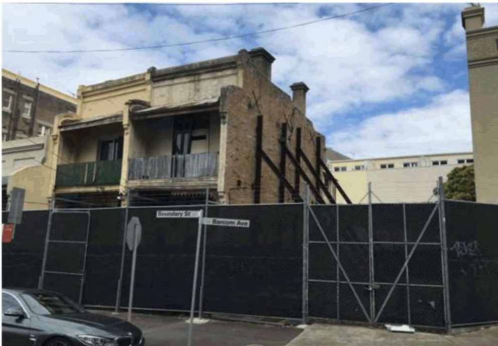
Figure 4: Existing dilapidated double storey terraces at 196-200 Boundary Street (source SJB)
