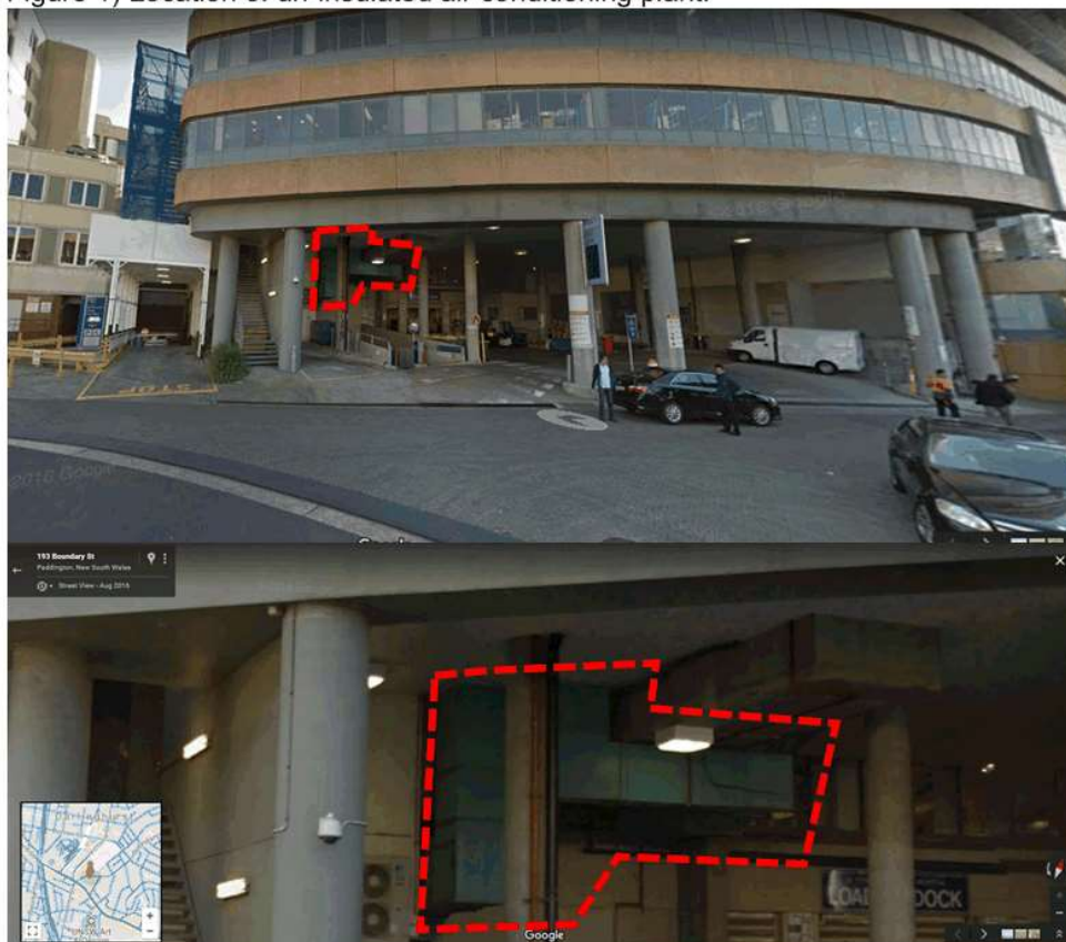
Figure 1) Location of un-insulated air conditioning plant.
