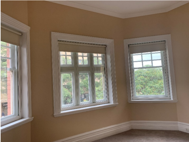
Figure 76 – First floor, timber-framed bay window in south-western room (all windows have later addition secondary frame for acoustic screening).
