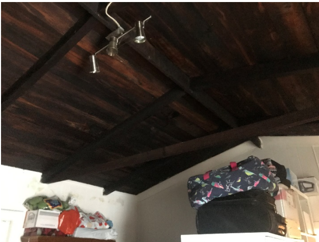
Figure 47 – Roof top apartment - timber roof structure with exposed stained beams and lining.
