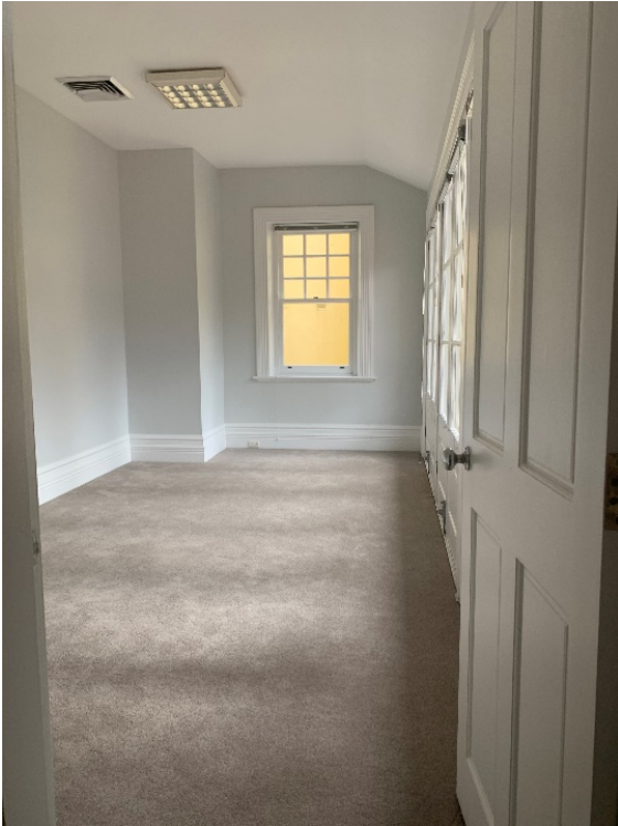
Figure 84 – First floor, north-western room with pitched roof – former verandah – and later addition, plasterboard ceilings and a/c vents.
