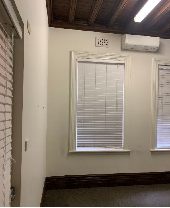
Figure 121 – Timber architraves and sills to windows in room at south-eastern portion of ground floor.
