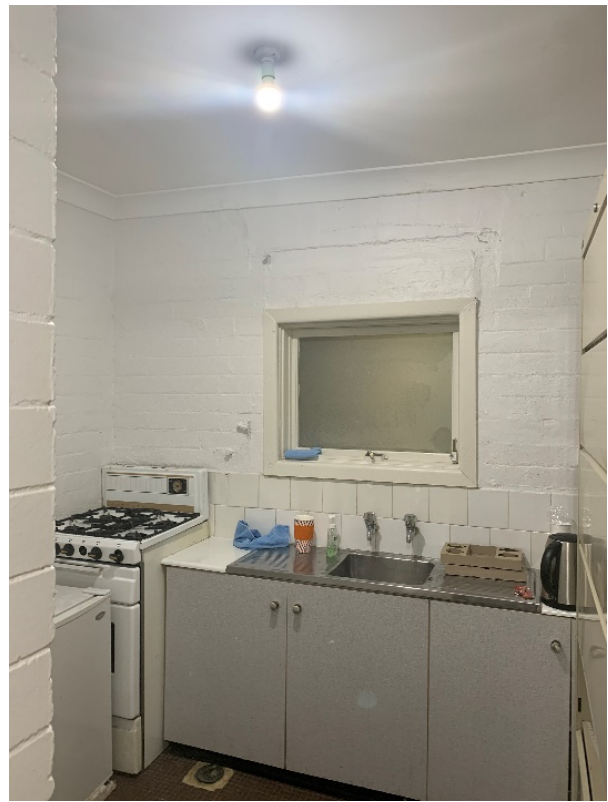
Figure 126 – Kitchen within secondary tenancy at northern wing of ground-floor. Painted face brickwork walls.
