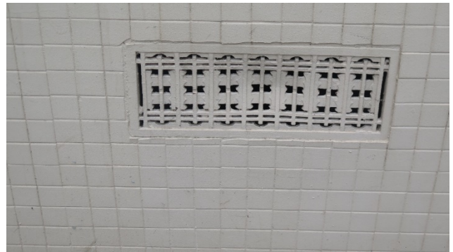
Figure 17 – Decorative air vent set into tiled wall finish
