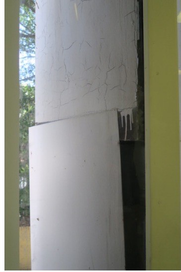
Figure 41.0, West facing louvres showing junction between metal plates, which needs re-fixing. Bronze finished stainless steel sheeted louvres have been painted white, at least 20 years ago. Removal of paint and restoration of original finish should be investigated.
