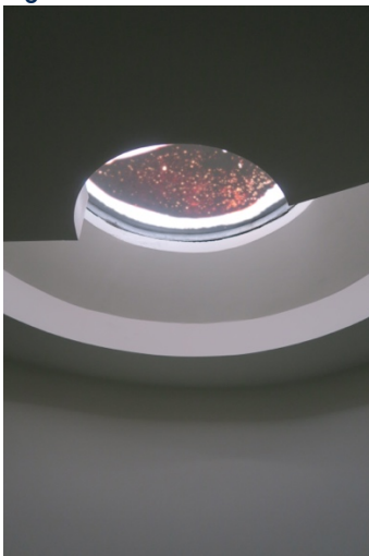
Figure 30.0, The original Perspex dome above the stair needs cleaning.
