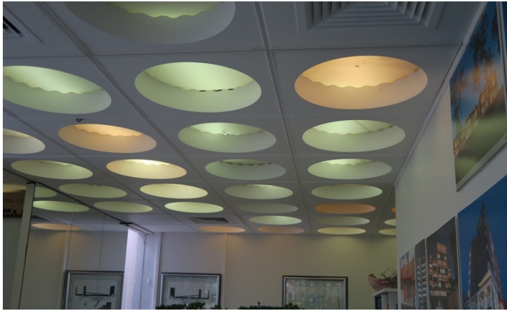
Figure 32.0, The special ceiling system devised by Gruzman which both lit the spaces and acted as a giant plenum for the air-conditioning system. Note that some new AC registers have been added.
