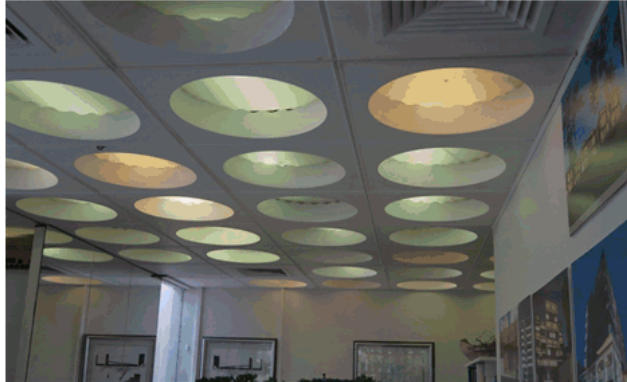
Figure 32.0, The special ceiling system devised by Gruzman which both lit the spaces and acted as a giant plenum for the air-conditioning system. Note that some new AC registers have been added.
