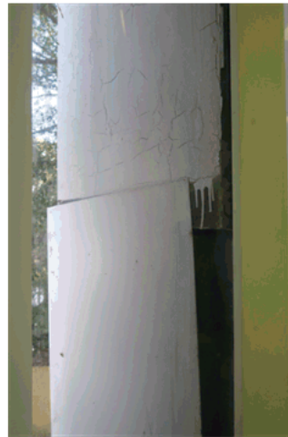
Figure 41.0, West facing louvres showing junction between metal plates, which needs re-fixing. Bronze finished stainless steel sheeted louvres have been painted white, at least 20 years ago. Removal of paint and restoration of original finish should be investigated.
