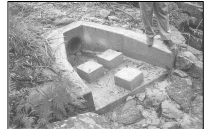
Photograph 2 Typical energy dissipater structure
