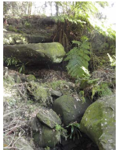
Magney Street drainage line
