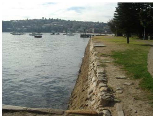
No beach access for launching kayaks (seawall)
