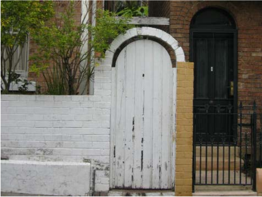
View 8: View of timber gate with masonry surround to side access of no. 33 Dudley Street Paddington, located within the street front zone and forming part of the principle elevation.
